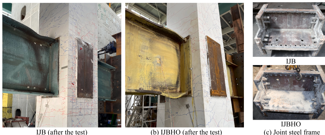
Fig. 8. Damaged state of specimens after the test: a) IJB, b) IJBHO, and c) joint steel frame.
